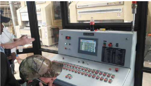
The control room of all the ginning equipment
